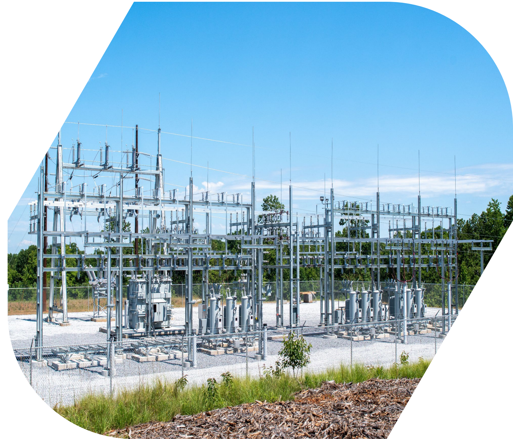
Aycock School Substation
